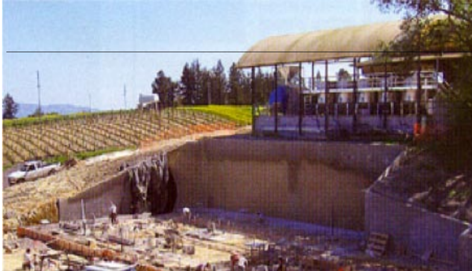
New fermentation building under construction. Direct access to the wine cave can be seen in the lower left had corner. The existing winery is higher on the hill. Below, a section of the caves under the canopy buildings.
